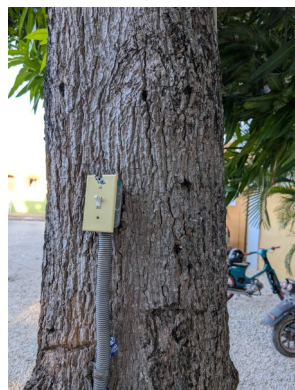
Who need an electrical post when you have a tree?
