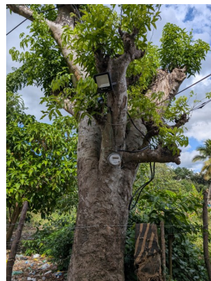
Electrial meter in a Bateye
